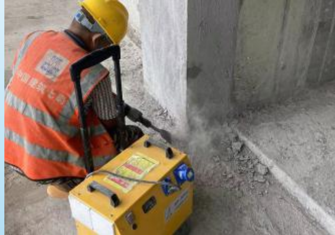
Power for renovation works
