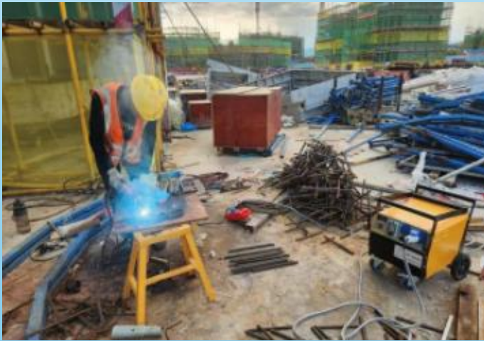
Power for construction works
