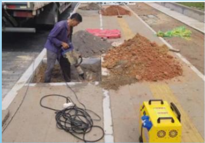
Power for municipal maintenance
